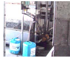
Cooling tower found bleeding to a storm water drain
