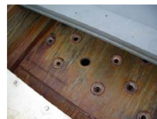
Missing cooling tower spray nozzles
