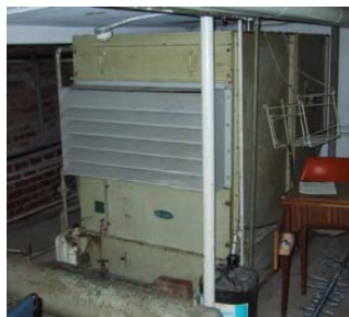
Absence of water treatment
