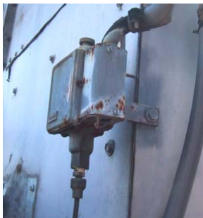
Control equipment not operational
