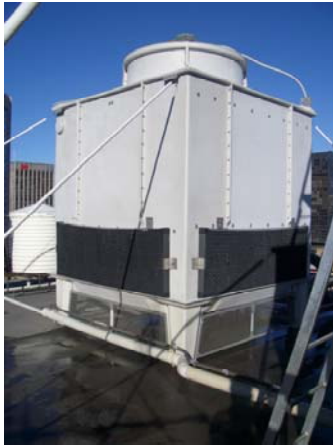
Significant water losses – water 'blown' out of the tower
